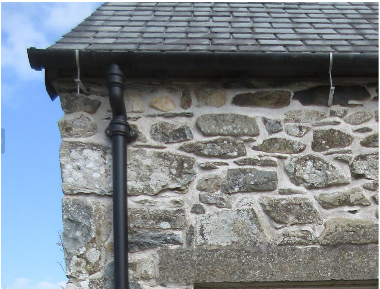
Photograph showing coated aluminium guttering painted black, or could be painted to match the windows. The guttering is attached with rise and fall brackets spiked directly to the wall.
