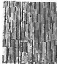
Dwarf wall clad with rustic copper stone to co with the surrounding landscape and environment
