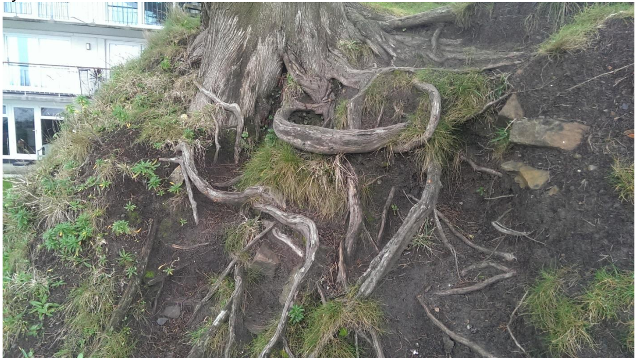
Appendix I – Significant roots exposed – no grass present to suggest dynamic erosion
