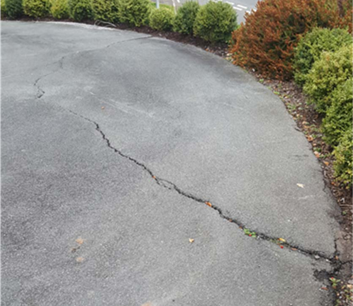
Image 9 - Crack visible in driveway – Tree is located to the right of the image.
